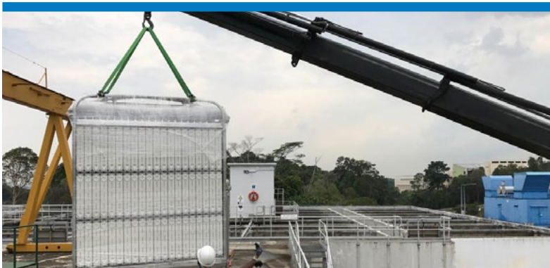
Replacement of Ultrafiltration Membranes and Addition of Membrane Cassettes at Choa Chu Kang Waterworks
