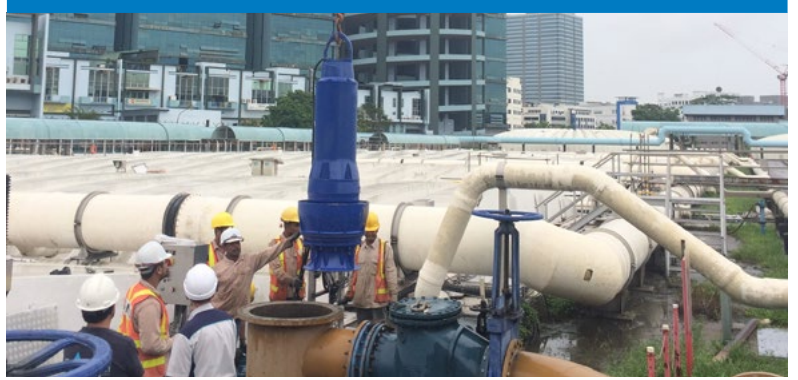
Servicing and Maintenance of Screening, Sludge, Grit and Related Equipment at Ulu Pandan Water Reclamation Plant
