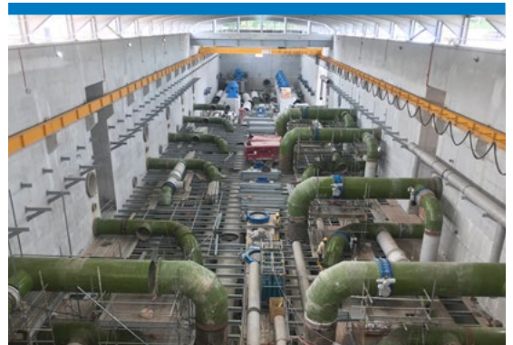
Process Upgrading at Choa Chu Kang Waterworks - Ozone and Biologically Activated Carbon Facilities
