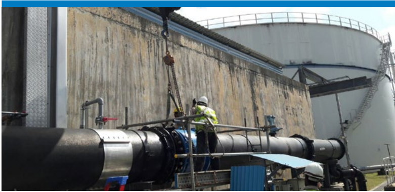
Supply, delivery, installation, commissioning and maintenance of Process Equipment at Kranji NEWater Factory
