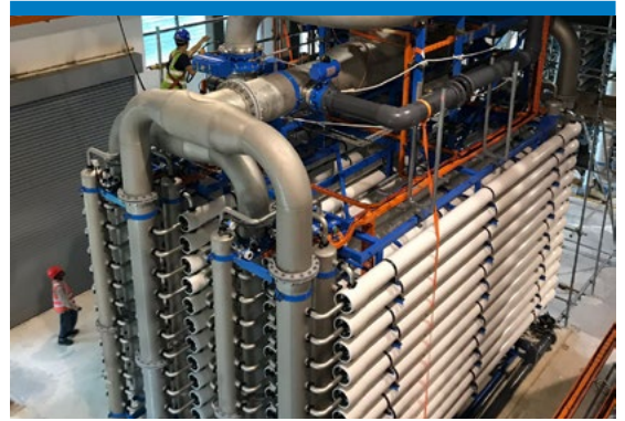
Supply, delivery, installation and commissioning of Membrane Train at Lower Seletar Waterworks
