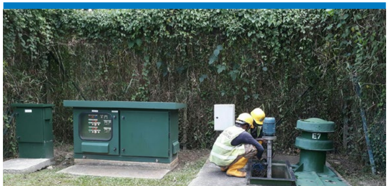
Operations and Maintenance of Lorong Halus Wetland Treatment System and Leachate Collection System
