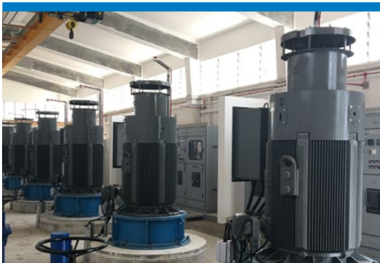
Replacement of Pump Sets, Associated Auxiliary Equipment and Pipelines at Jalan Eunus Booster Station
